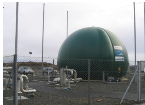
Figure 10 – Example of Biogas storage system
