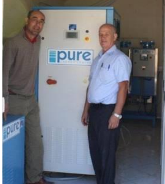
Figure 2.3 – A hydrogen electrolysis unit as installed 3
